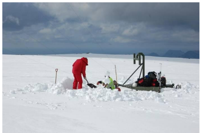
Figure 4-5: Accessing power system in a remote location. The whole 2.5-meter high container apart from the air inlet to the engine has been buried. Photo credit: Lars Tallhaug, Norway
