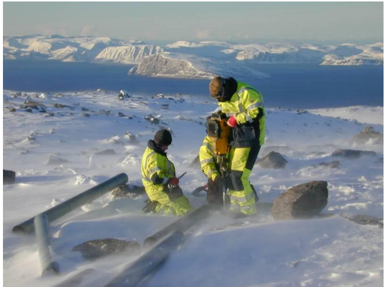
Figure 8-3: Work in extreme and cold climates requires special equipment, increased focus on personnel safety and expanded planning. Photo credit: Lars Tallhaug, Norway
